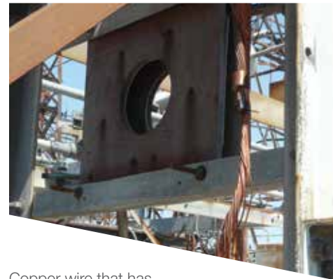
Copper wire that has been tampered with at an electrical substation in Ontario.
