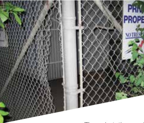
The substation yard where the thief broke in, attempting to steal copper. (Source: EPCOR Utilities Inc.)
