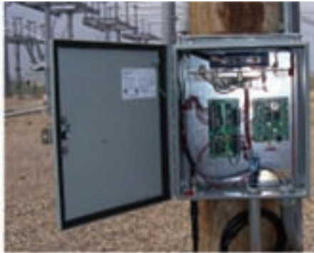
Figure 6 – TRM Controller at Lyon County Substation (LYC)
