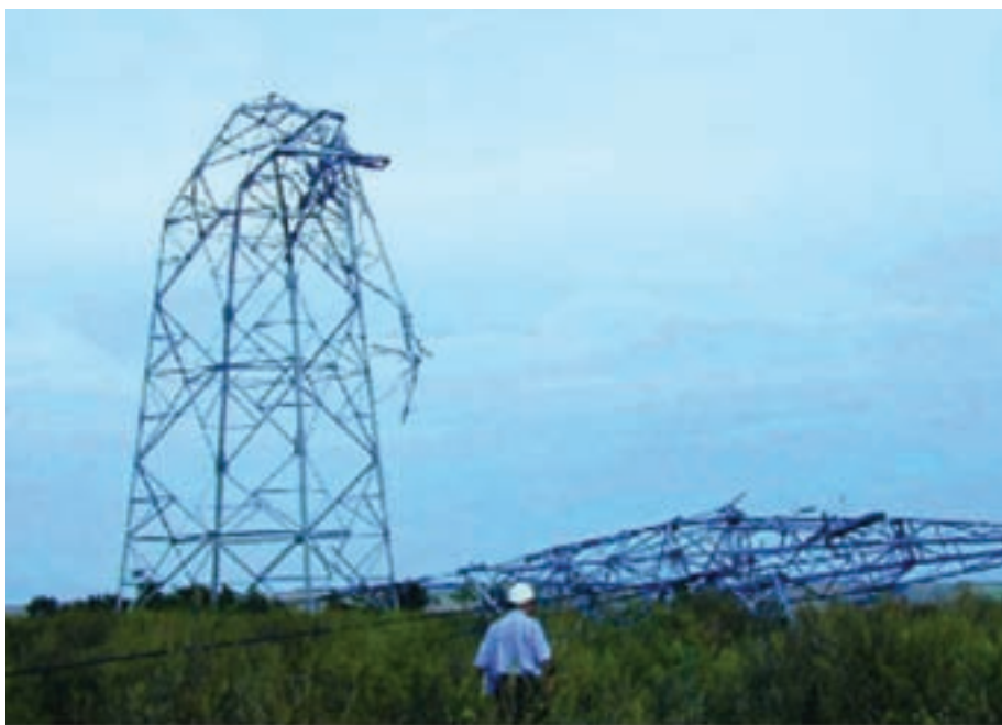
Tower failure due to high winds.
