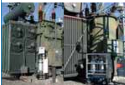
Figure 4: Dehydration Unit D1 (left) and Decontamination System Mark II (right) Installed on 60kV Field Transformers
