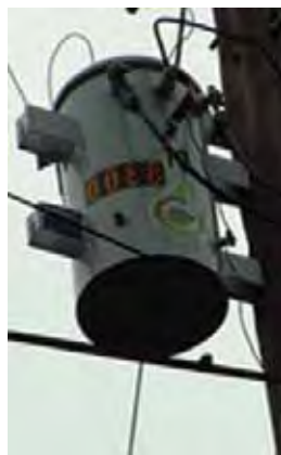
Transformer filled with new soy-based fluid.
