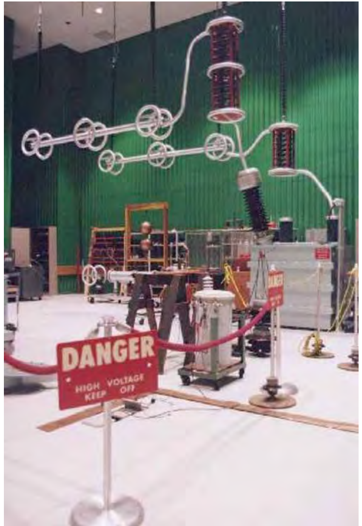
Figure 1. View of the 250 kV transformer, current limiting resistors and high voltage buses.
