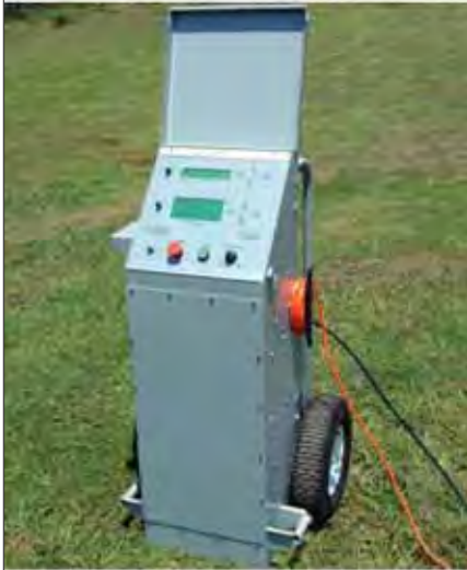
VLF Cable Testing
