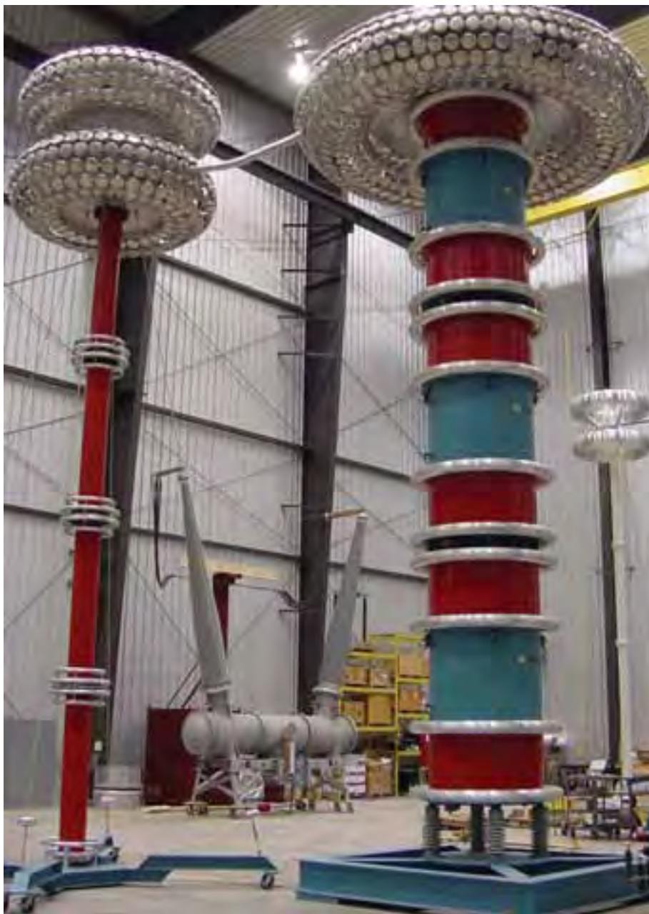
The AREVA T&D high voltage test lab in Charleroi, PA will be featured during Tuesday's Factory Day at the Circuit Breaker Test & Maintenance Conference in October.
