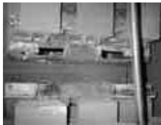
Figure 1: 3000 amp 600 volt bus fault
