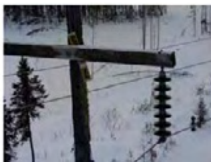
115 KV Suspension string.
