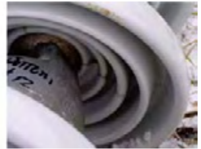
Cracked insulator skirt.
