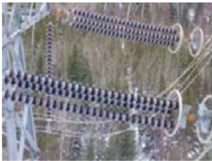
500 KV Dead-end string.
