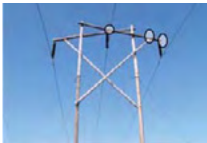
230 kV pole structure showing suspect locations of high failures
