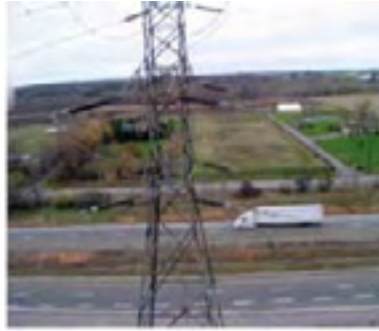
230 KV Dead end tower
