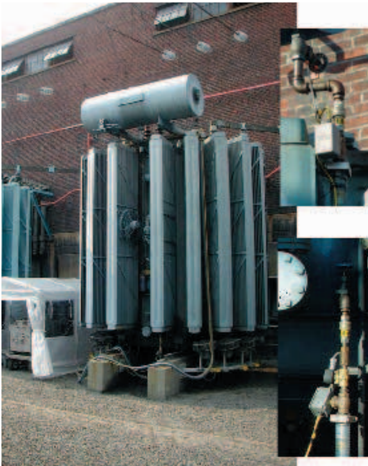
Figure 4. Dryout site example. Rectifier transformer, 9300 kVA, 13.2kV/.624kV, 16,000 litres have been dried. Observe the hydraulic connection at the bottom of the main tank and the expansion tank.
