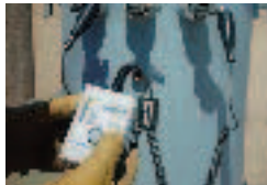
Checking transformer condition (Photo: Hastings)
