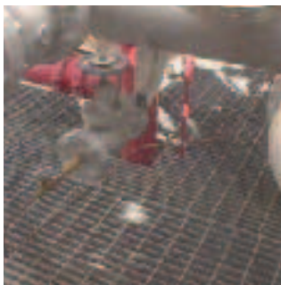
Figure 2A: Transformer supply valve
