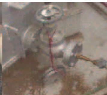
Figure 2B: Transformer return valve
