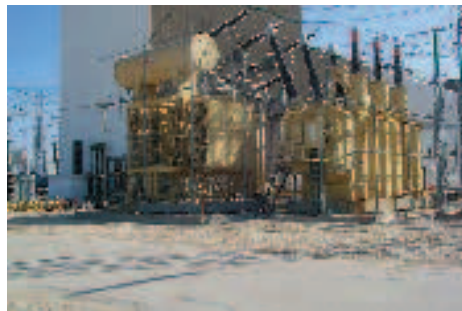
Before installation: Note old radiator coolers in block with poor airflow.
