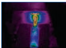
Bad bus-breaker connection
