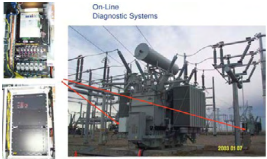
Figure #16: Case #5, Transformer Photos
