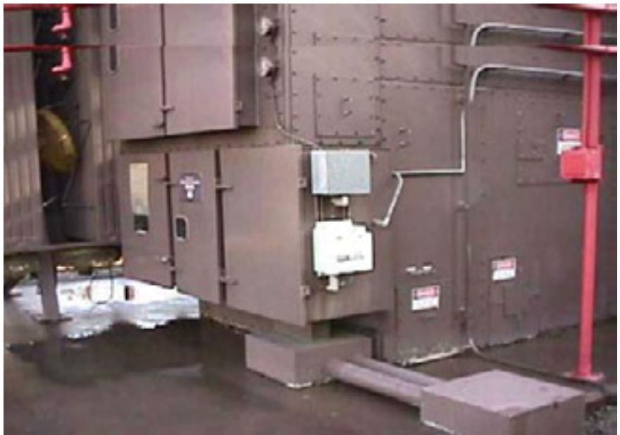
Figure #19: Case #7, LTC Sensor Installation
