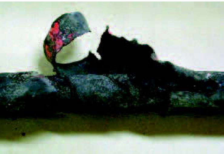
Corroded metal shield causing failure from outside in
