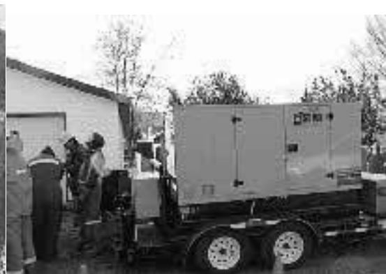
Figure 5: Mobile generator provides temporary power, as cable segment is de-energized
