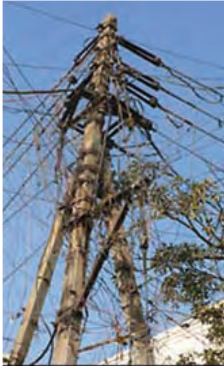
Powerlines can more resemble Christmas trees covered in tinsel as people attach their own lines to steal electricity.
