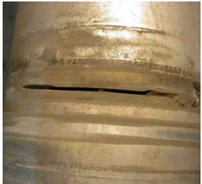
Figure 2 Damage caused by arcing
