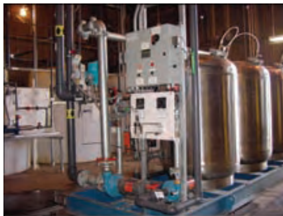
Sonitec uses a centrifugal sand filter to process water cleaner.
