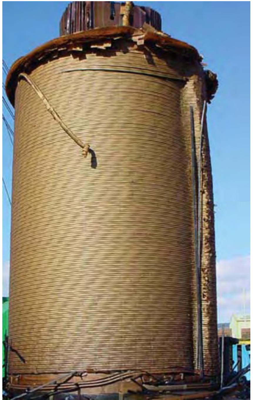
Figure 9 Winding showing significant buckling
